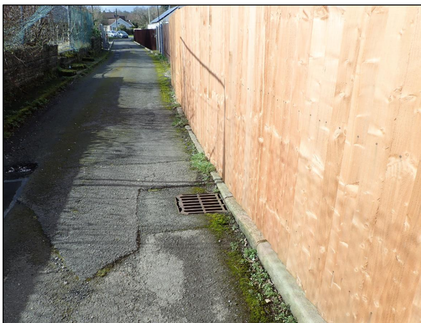
Figure 5: Dropped kerb and highway gully at Meadow Lane, to the rear of the impacted properties at Beacons View (image captured by RCT's Flood Risk Management officers on 26/02/2020)
