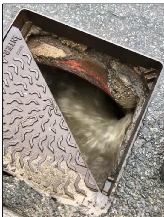
Figure 10: Photo of 'Manhole 1' surcharging during Storm Jorge (captured by RCT's Flood Risk Management team on 28 th February 2020)
