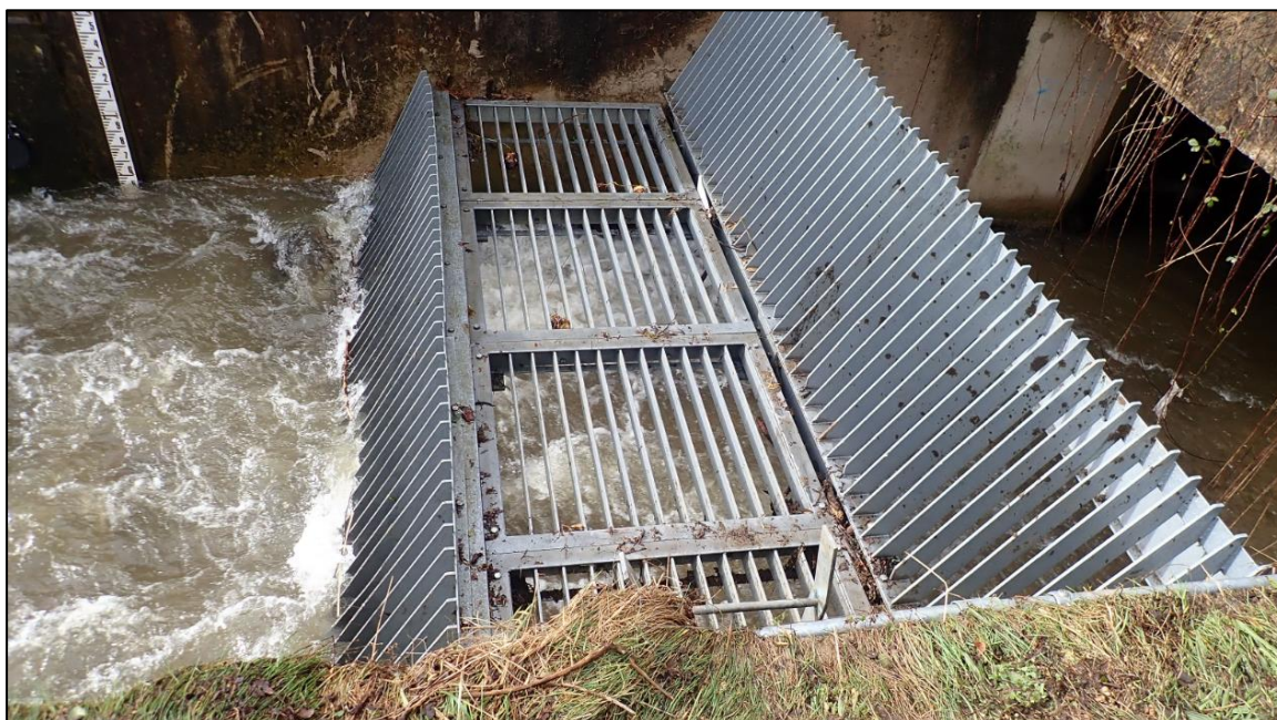
Figure 17: Nant Cae Dudwg culvert inlet (captured by FRM officers on 17 th February 2020)
