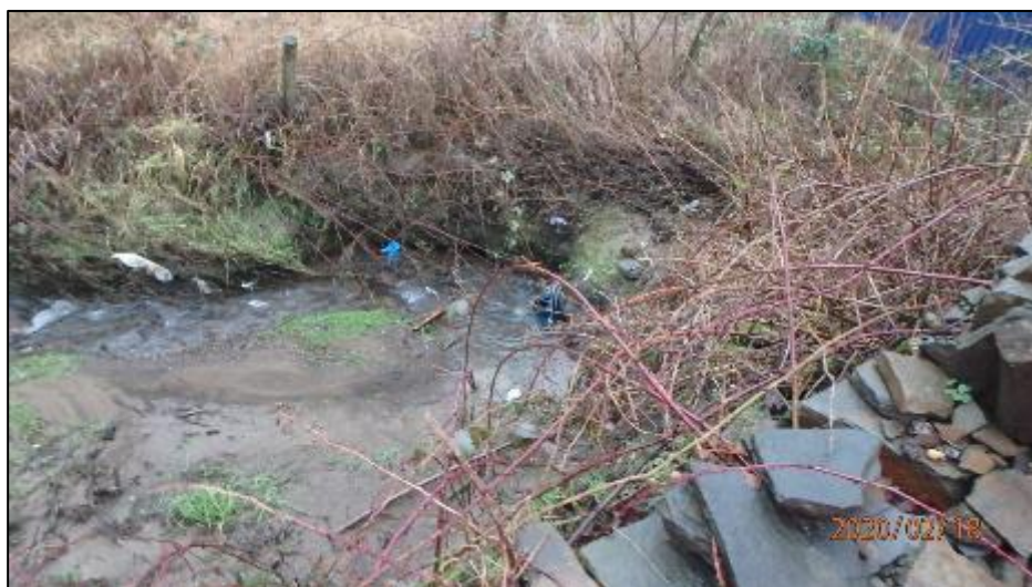
Figure 5: Evidence of submerged 'Culvert Inlet 1' which surcharged during Storm Dennis (captured by RCT's Flood Risk Management team on 18 th February 2021)
