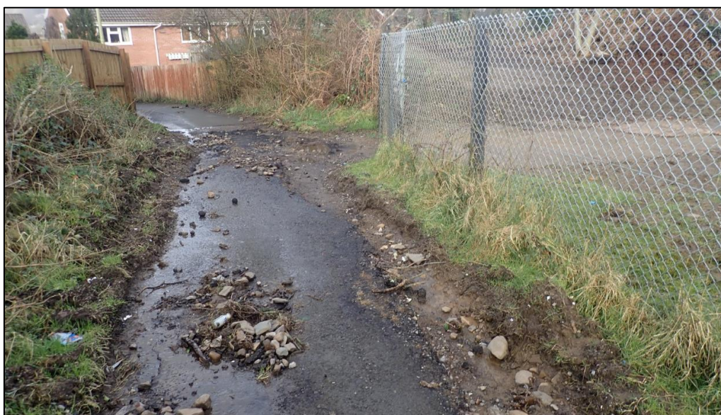
Figure 12: Evidence of deposited debris and damages to the bottom of the path looking down towards Brynderwen. Overland flows were observed flowing through land to the right behind the fencing (captured by FRM officers on 17 th February 2020).
