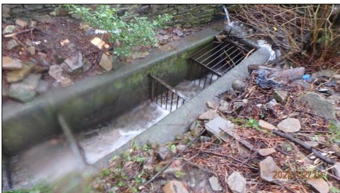
Figure 7: 'Culvert Inlet 3' to the rear of Dumfries Street which surcharged during Storm Dennis (captured by RCT's Flood Risk Management team on 19 th February 2021)
