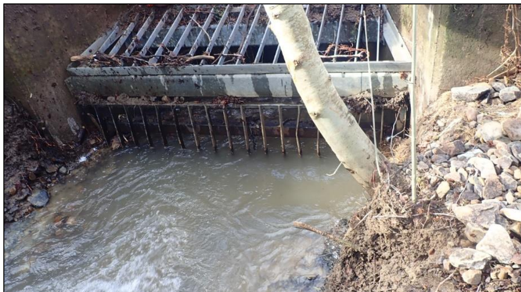
Figure 18: Culvert inlet to the rear of Heol Mynydd which surcharged during Storm Dennis due to blockages at the inlet (captured by FRM officers on 17 th February 2020 following clearance works)
