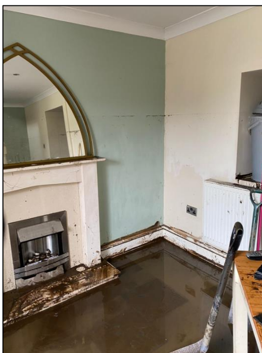
Figure 7: Water depth marks in a property at Cilfynydd Road following Storm Dennis (image provided by resident)
