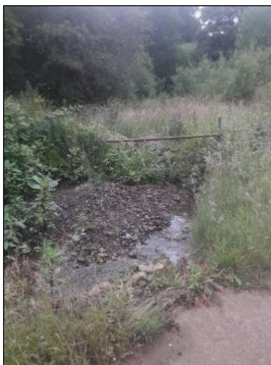
Figure 20: Image of debris accumulation within the unnamed ordinary watercourse channel upstream of 'Culvert Inlet 1' (Figure 4) (captured during CCTV operations on 30/06/2020)
