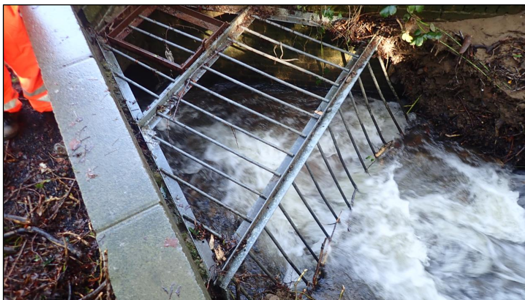
Figure 19: Ely Brook culvert inlet to the rear of Pontshonnorton Road which surcharged during Storm Dennis due to blockages at the inlet (captured by FRM officers on 17 th February 2020 following clearance works)
