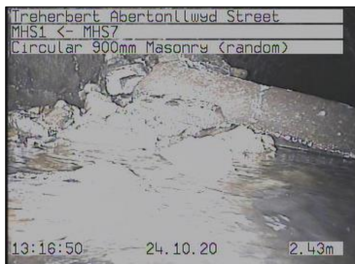
Figure 15: Internal view of 'Abertonllwyd Street Culvert Network 1' downstream of 'Manhole 1' (CCTV survey footage captured 24/10/2020)
