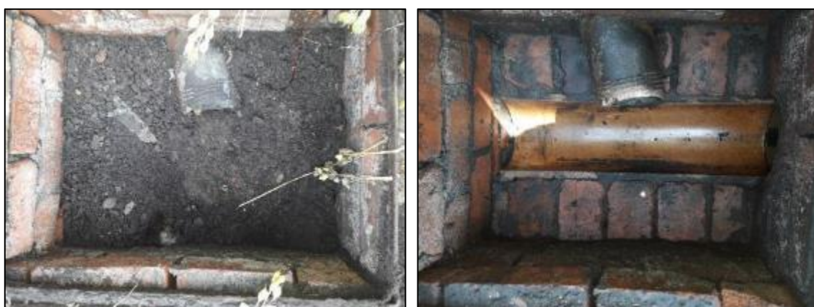
Figure 15: Photo of a manhole at Oxford Street captured before (left) and after (right) surveying and cleansing operations during June 2020
