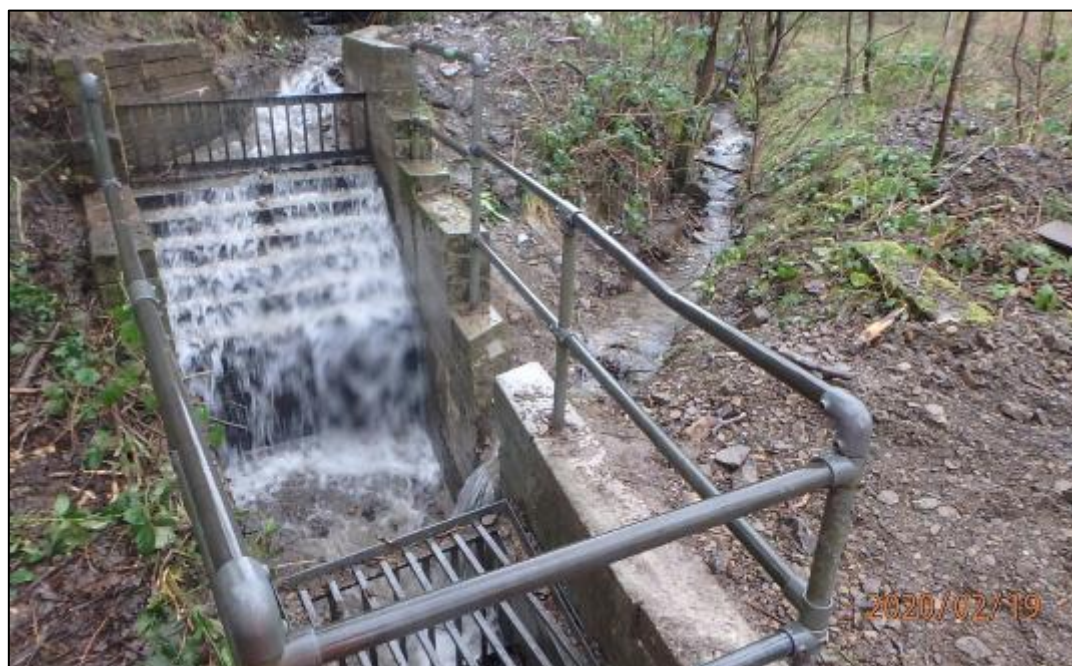
Figure 18: Photo of 'Culvert Inlet 6' captured by RCT's Flood Risk Management team following debris clearance post Storm Dennis (19/02/2020)
