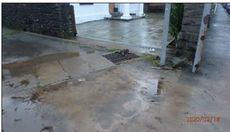
Figure 6: 'Manhole 1' located at Abertonllwyd Street surcharged during Storm Dennis (captured by RCT's Flood Risk Management team on 18 th February 2021)
