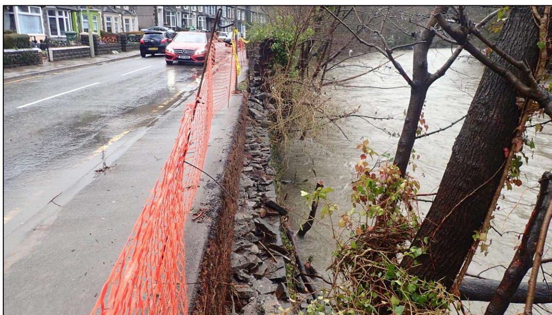
Figure 5: Collapsed river wall (NFD) on Berw Road following Storm Dennis (captured by RCT's Flood Risk Management team on 17 th February 2020)
